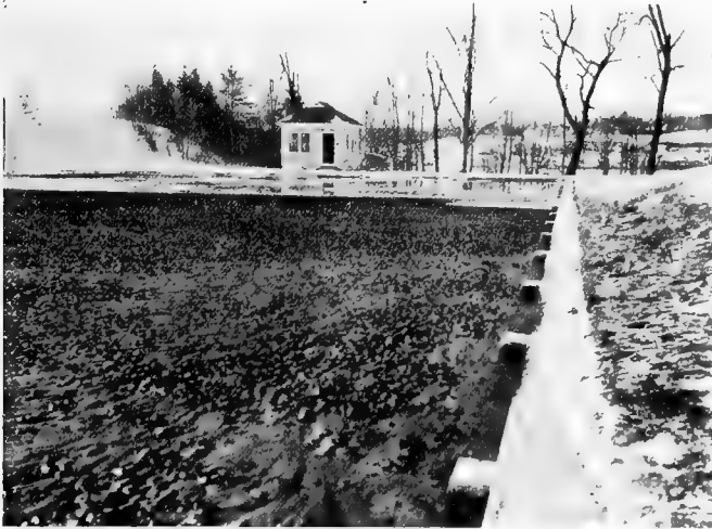
Fig. 50.—Stone bed of a sewage disposal plant.
